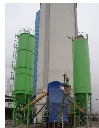
Fig. 3. The view of the tanks A and B in the factory in Konin (Poland)
