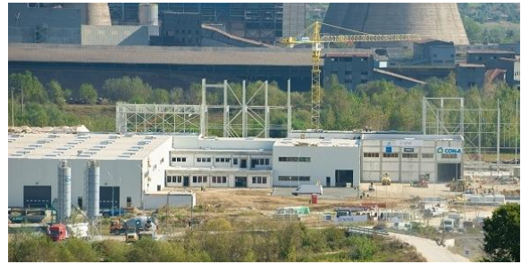
Fig. 1. A view of the ETEX Building Performance S.A. production hall in Turceni (Romania).
